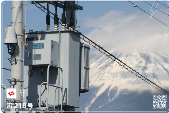
Fig. 3 Utility pole NFT card (Numa 218)
