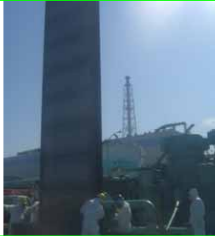
Sliding timber weir in seawater pump house for auxiliary equipment cooling was already installed (Unit 2) (Completed by May 24)
