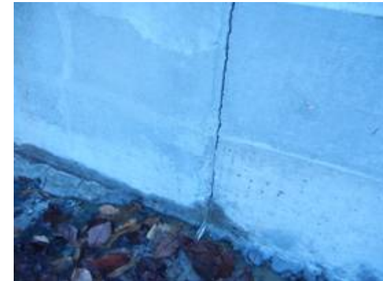
Status of leaking point
