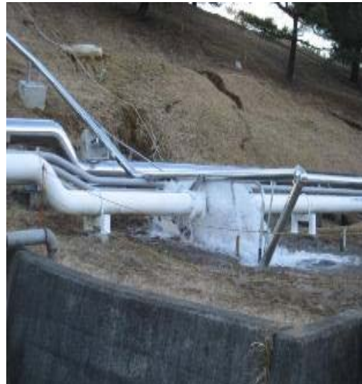
Leak from the disaster prevention piping for transformers
