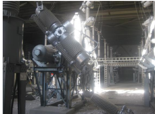
Part of the circuit breakers, damaged in the tsunami, in the switching station fell off.
