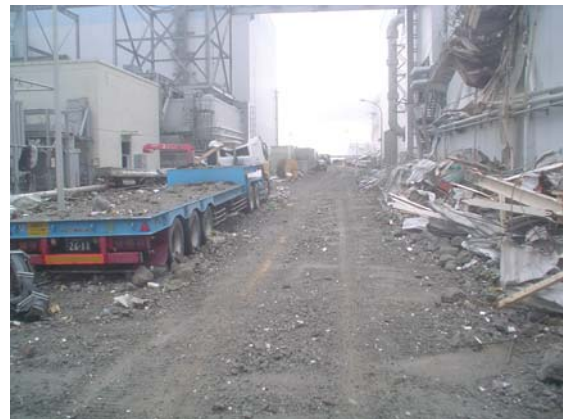
Units 3&4 transformer area after a trailer and debris were cleared aside (photo taken on a later day)
