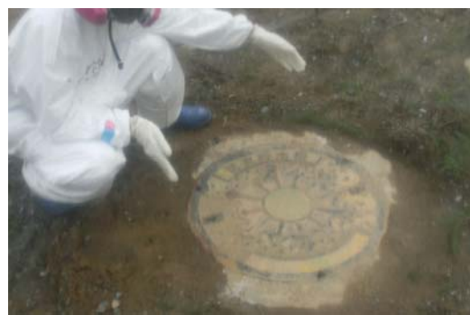
Intake cover of a fire protection tank
