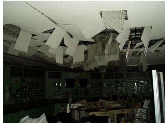
Main Control Room after the explosion
