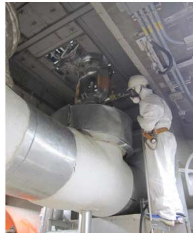
RHR injection valve fixed on a pipe of approx. 60cm diameter (Unit 5, with light)
