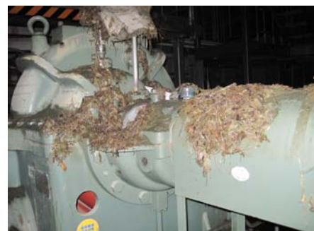
Submerged seawate pump (the photo was taken at a later date)
