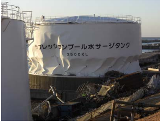
Tank deformed in the tsunamis (One of the tanks in the photo above)
