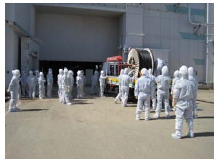
Preparations for laying temporary cable (photo of work conditions at a later date)
