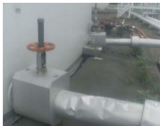
Outlet valve of a filtrate tank
