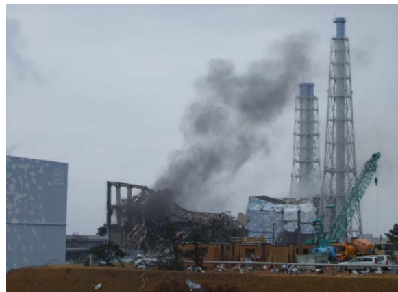
Appearance of Unit 3 immediately after the explosion (Photo taken on March 21, 2011)
