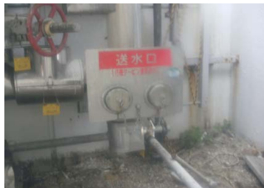
Outlet of Fire Protection System of Unit 1
