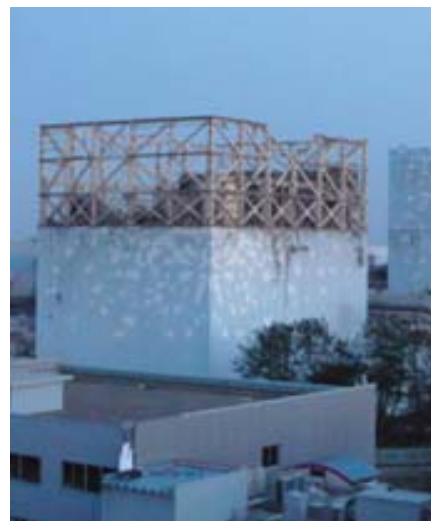
Reactor building of Unit 1 after the explosion
