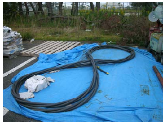
The cable in the photo, weighing 90kg, is approx. 15m long. A cable at least ten times longer than this one was used to restore the power supplies of Units 1 and 2.
