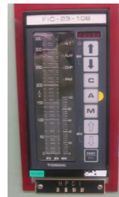
HPCI flow instrument controller (FIC) (Photo taken on a later day)
