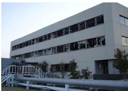
Main office building with shattered windows in the blast
