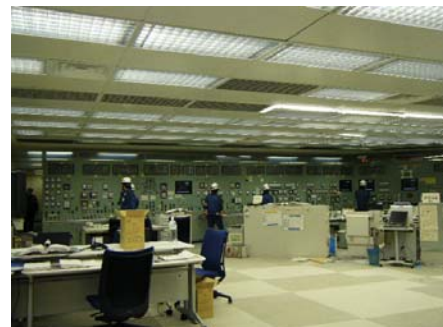
Main control room after tsunami arrival
