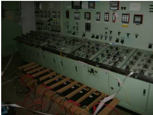
Instruments connected to temporary accumulators as power supplies
