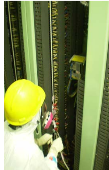
Rear side of the control panel (Photo with light taken on a later day)
