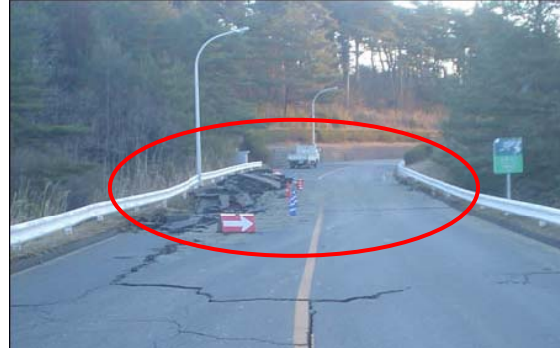
Damage to the access road to Units 5 and 6 (After restoration. Some pavement on the other side was stripped to obtain ballast and gravel to fill in bumps on the other side of the road.)
