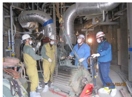
Pump motor recovery work (photo of work conditions at a later date)
