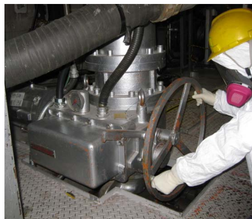
Image of rotating the RHR injection valve (Unit 5,
