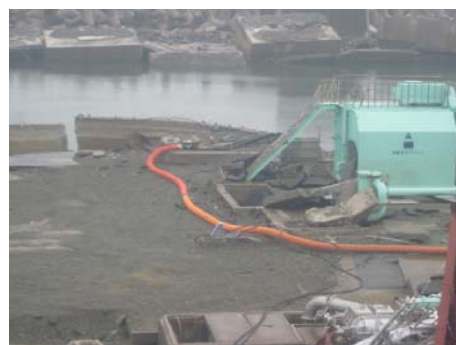
Underwater pump installation conditions (arrangement done at later date)
