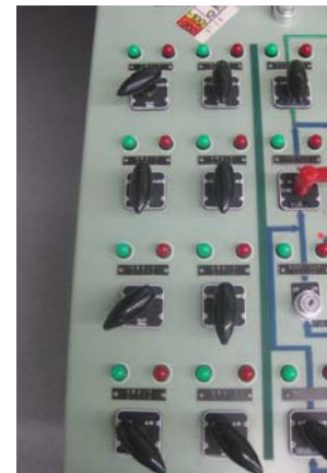
SRV control panel (photo taken
