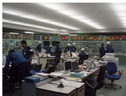
Unit 5/6 main control room: Unit 6 side
