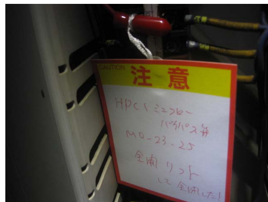
HPCI control panel
