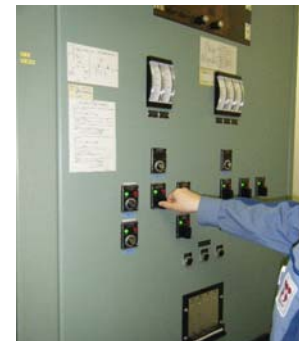
Valve operation at main control room AM panel (photo of work conditions at a later date)
