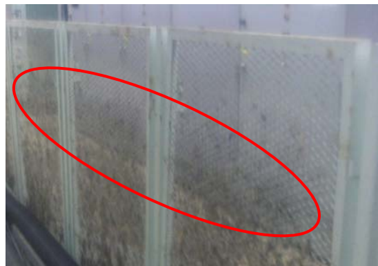
State of M/C on the first floor of the Unit 1 Turbine Building
