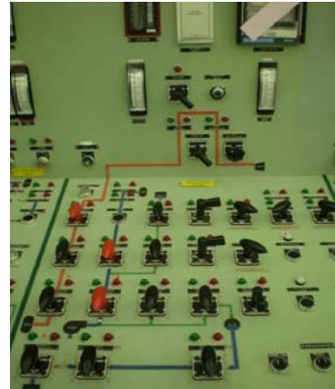
HPCI control panel (photo taken on a later day) All the status indicators went out on the day.
