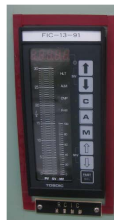
RCIC flow rate controller (FIC) (Photo taken on a later day)
