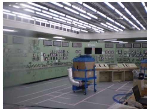
Main Control Room of Units 1 and 2 (photo taken later)
