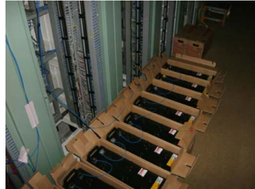
Ten 12V batteries in serial connection (Photo with light taken on a later day)
