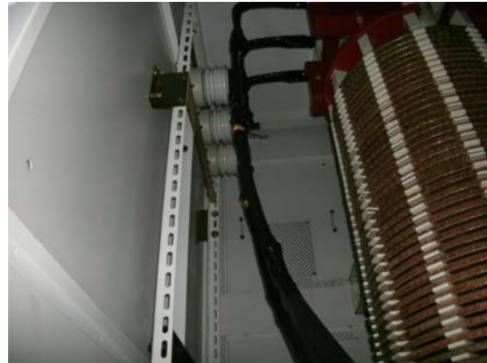
Connecting a 3-line cable to the power supply panel. The 3-line cable terminals are fixed with bolts and rolled up in insulation tape.
