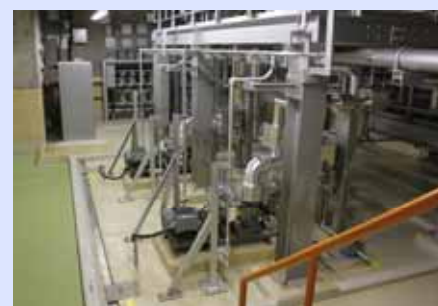
Current condition of the heating steam condensate Water transfer pump in Unit 3 T/B 2nd basement (Photo taken on May 24, 2012)
