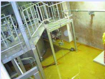
Flooded condenser room in Unit 1 T/B basement (Photo taken on March 20, 2011)
