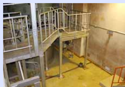
Current condition of the condenser room in Unit 1 T/B basement (Photo taken on May 24, 2012)
