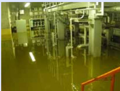
Flooded heating steam condensate water transfer pump in Unit 3 T/B 2nd basement (Photo taken on March 19, 2011)
