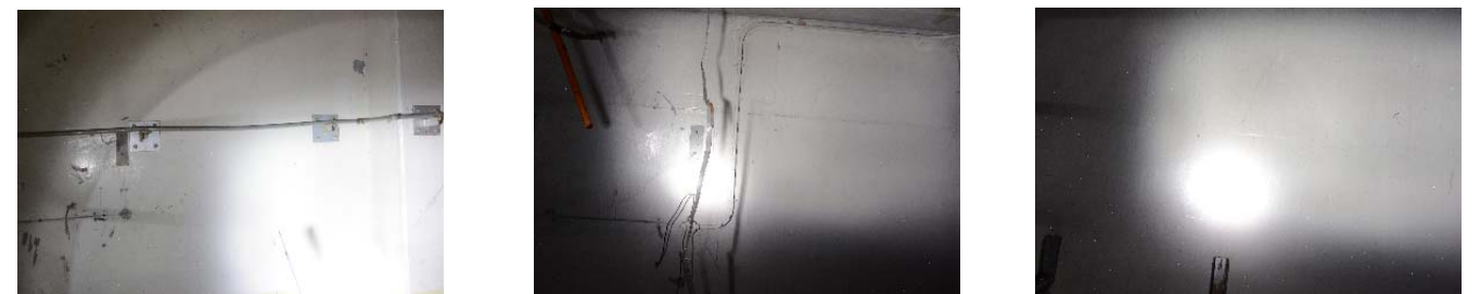
Figure 3: Unit 1, on the west-side walls facing the equipment hatch (center part) (from left, 4 th , 3 rd and 2 nd floors)
