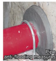
Pipe anti-flooding measures
