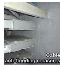
Cable anti-flooding measures
