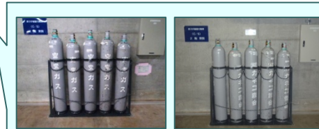
Backup nitrogen cylinders (5 cylinders x 2)/ 1 plant
