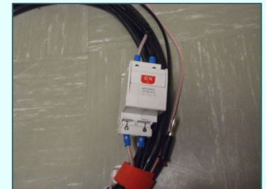
Provisional control switch and provisional cable
