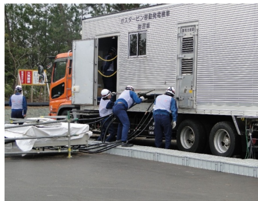
Training scene: Supplying power using GTG
