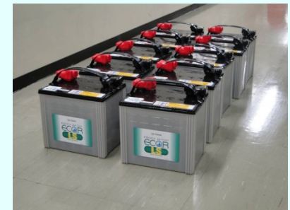
Auxiliary storage batteries
